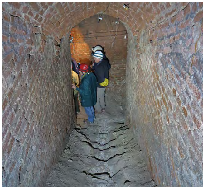
Entrance passage showing degraded steps at Graincourt muche
